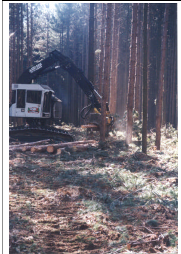
Figure 9 The Division of Forestry will continue to encourage the use of the recommended harvesting technology (known as cut-to-length) on State Forests as well as private lands. The pictured machine conducted a harvest at Maumee State Forest in early 2001.
